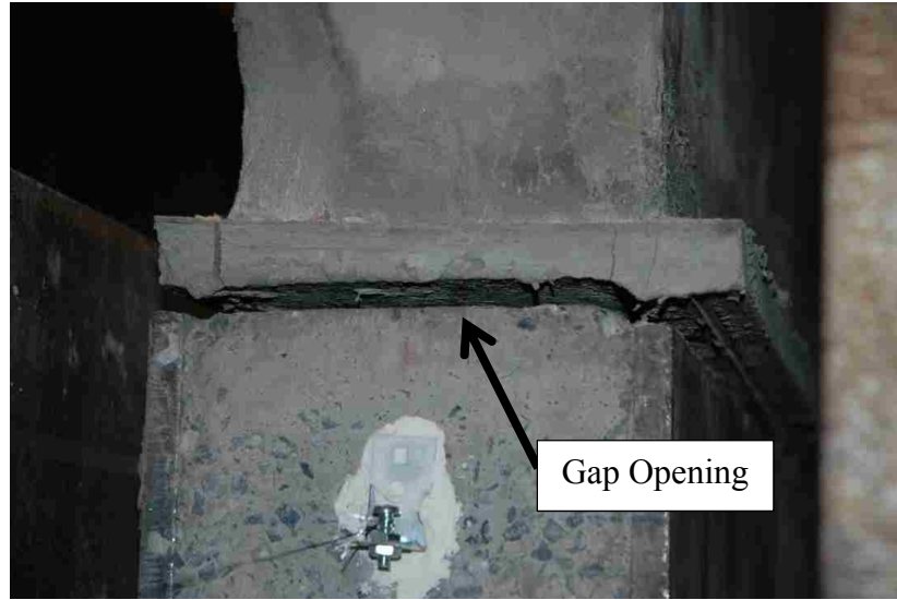
Figure 5-24 - Gap Opening at Joint between First and Second Panels 2% Roof Drift (Westward Loading)
