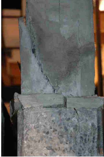
Figure 5-4 - Damage Event 1 - Top Corner of Plate-Confined Panel (West Side)
