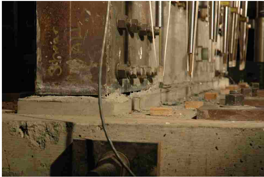
Figure 5-5 - Gap Opening at 0.75% Roof Drift (Eastward Loading)
