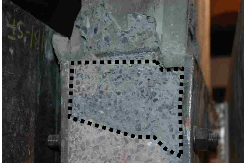
Figure 5-6 - Area of Concrete Removed During 1.0% Cycles (West Side)
